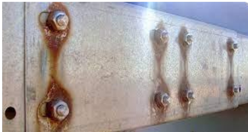
Figure 1: Effects of Corrosion on Mild Steel (Marder, 2018)
